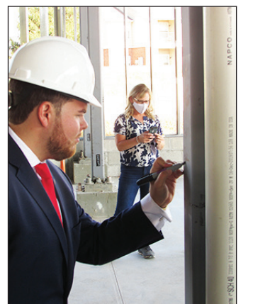
City-County Council member Paul Annee signs beam that is in place at West Perry Branch library interior.
