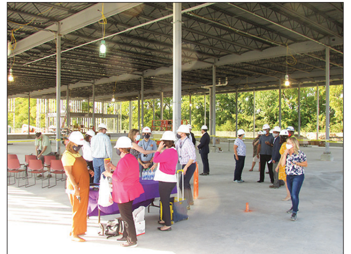
(SOUTHSIDER VOICE PHOTO BY AL STILLEY) V.I.P.'s and Indianapolis Public Library representatives enjoy refreshments on the spacious floor of the West Perry Branch library that is under construction.
