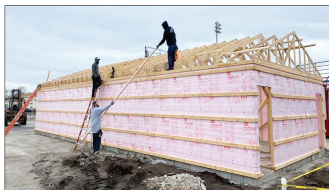
(SUBMITTED PHOTO) Workers at the Indianapolis Speedrome continue to make improvements at the near-southeastside race track. A new and spacious building or concession sales and men's and women's rest rooms is going in behind the third-turn bleachers. The new building is among the many improvements that have been made under the ownership of used-car dealership owner Dennis Garrigus, who has improved spectator and participant amenities at the track at Kitley Avenue and Brookville Road. Preparations are under way for the track's 79th season.
